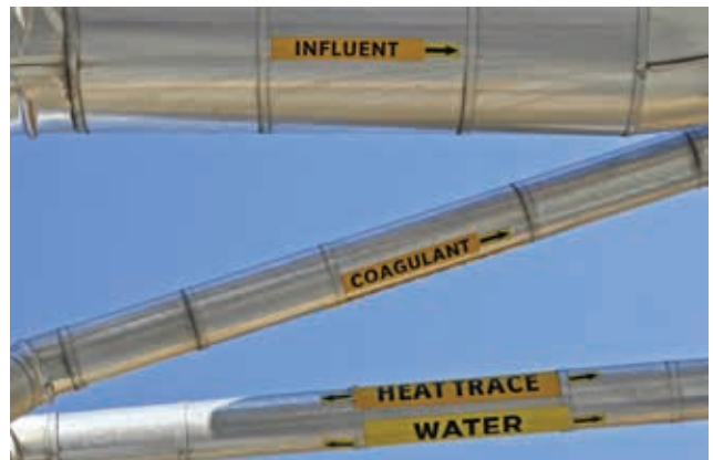
Pipe marking in industrial environments
